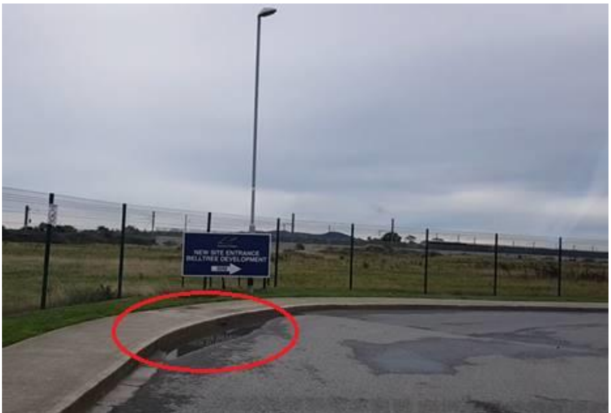
Figure 7: Ponding in carriageway
