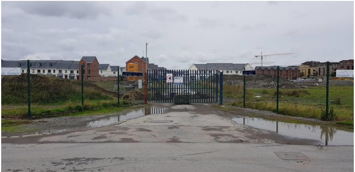
Figure 6: Ponding at Junction
